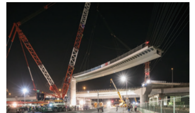
Construction work of Nagoya-daini-kanryo Expressway Tobishima Junction C Ramp Bridge and other 3 Bridges (Steel Superstructure) (NEXCO Central)
