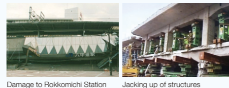
Damage to Rokkomichi Station Jacking up of structures
