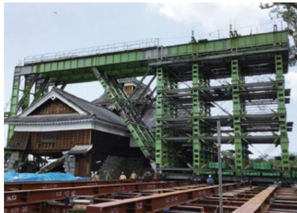
Collapse prevention equipment
