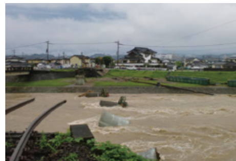
The damage to the Kagetsugawa Bridge
