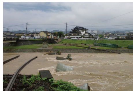
The damage to the Kagetsugawa Bridge
